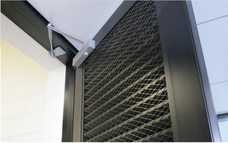
Door with MAL 40mm Single Bank and integrated vermin guard - St Cuthberts School, Centennial Pool Complex, Auckland.
