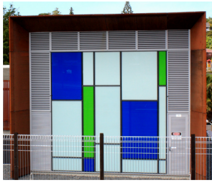
Door with MAL 40mm Single Bank & curtain wall with integrated MAL 100mm Single Bank - Vector Substation, Auckland.
