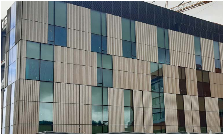
Taranaki Base Hospital Extension - unitised aluminium planking integrated into PW1000 High Performance Unitised Curtainwall.
