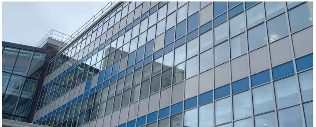
UOO Dental School, Walsh Building - PW1000 replicating the pattern and colour of the original 1960s design to maintain the connection to the iconic past facade
