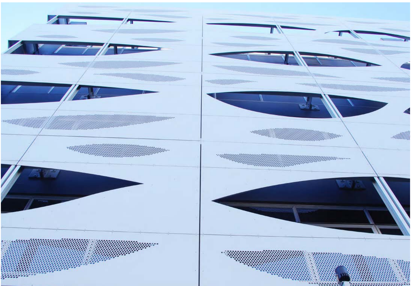
15 Huron Street, Takapuna, Auckland - Laser cut and perforated solid aluminium solar shade screens
