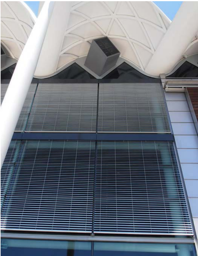
Viaduct Events Centre, Auckland - External Venetian blinds for solar and sight screening.
