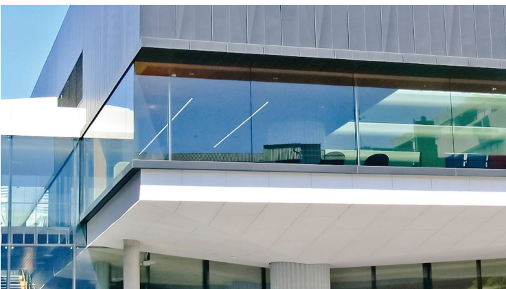
Victoria University Wellington, The Hub, Kelburn Campus - channel glazing to upper level
