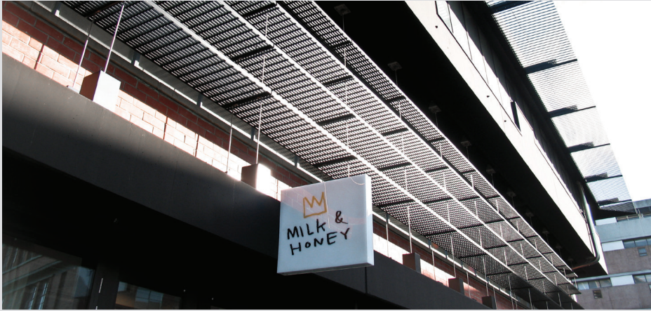
Shadetread™ installed to facade as external trafficable sunscreens - Victoria University, The Hub, Kelburn Campus
